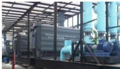
The largest power generation capacity of distributed energy system in China
